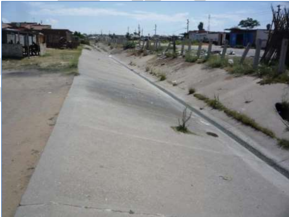
Figure 19, position 5: View south (upstream) from further down the concrete-lined canal than Fig. 18, showing the incursion of temporary shelters, sales areas and litter along the edges. Note the impermeable road surface running alongside the canal and lack of any flow-reduction structures within the relatively steep canal.
