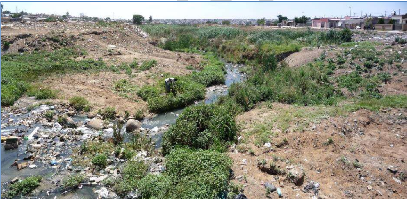
Figure 29, position 9: View east (downstream) where the K2 Tributary flows out from under the Glassnose Street crossing and constriction. Note the eroded bed and banks, and the degraded and transformed edges of the watercourse between the housing, with minimal marginal vegetation to protect and retain them.
