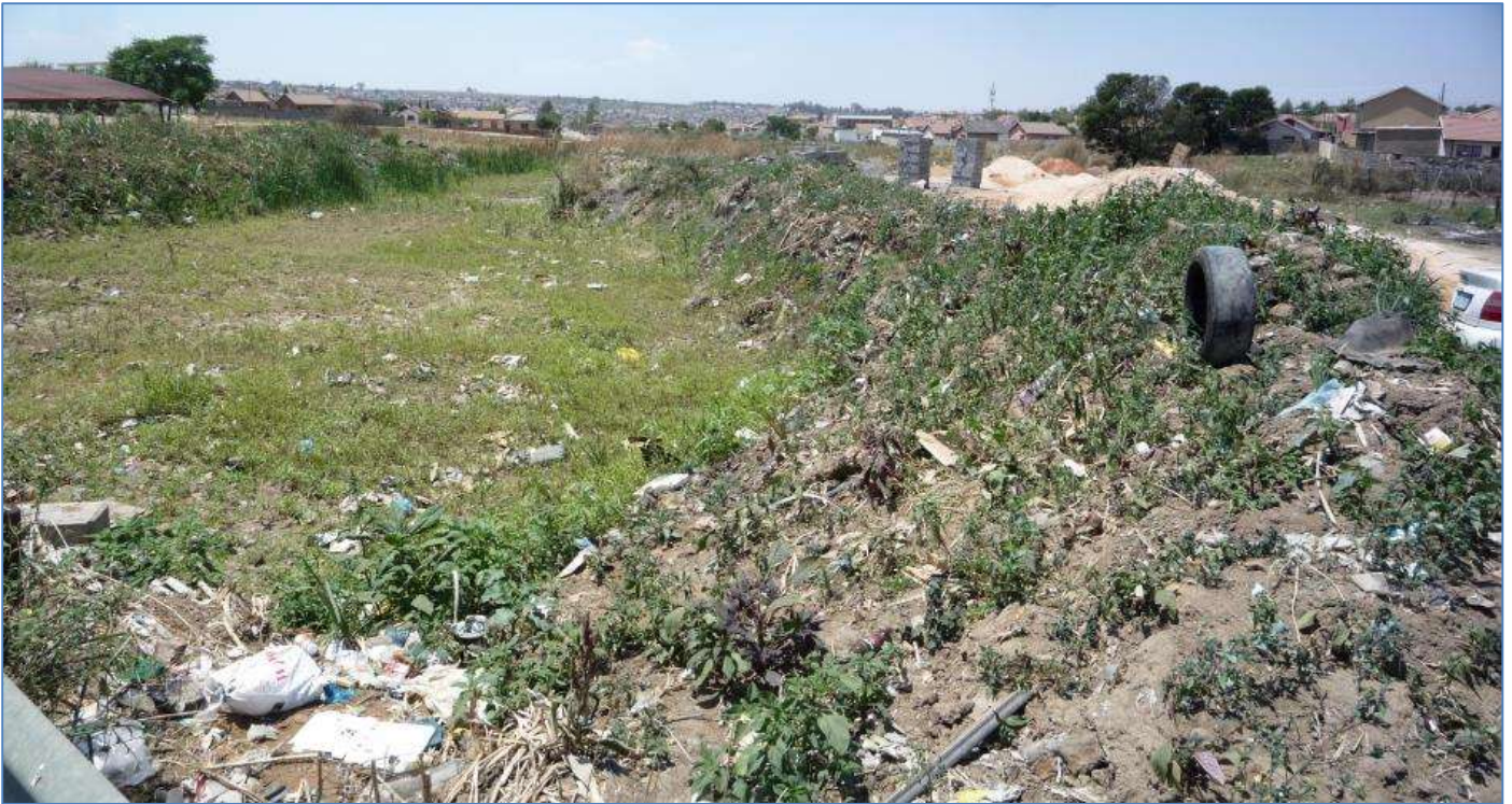
Figure 36, position 11: View northeast along the K2a Tributary below where it crosses Camellia Street, showing the narrowed and channeled drainage line with earth berms on either side, sited some distance from the nearest housing and presumably to protect it from flooding. Note the highly degraded secondary vegetation that has appeared, much of it alien species.
