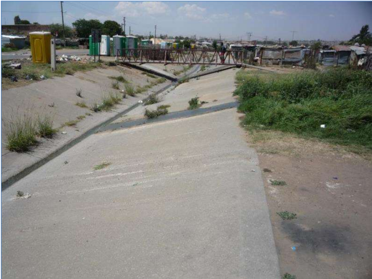
Figure 20, position 5: View north (downstream) from the same position as Fig. 19, showing weeds growing where runoff/seepage down a side street leaks into the canal, a pedestrian bridge across the canal, informal housing encroaching on the east (right) bank and portable toilets on the west (left) bank. Note the lack of any flow-reduction structures within the canal and its relatively steep gradient.
