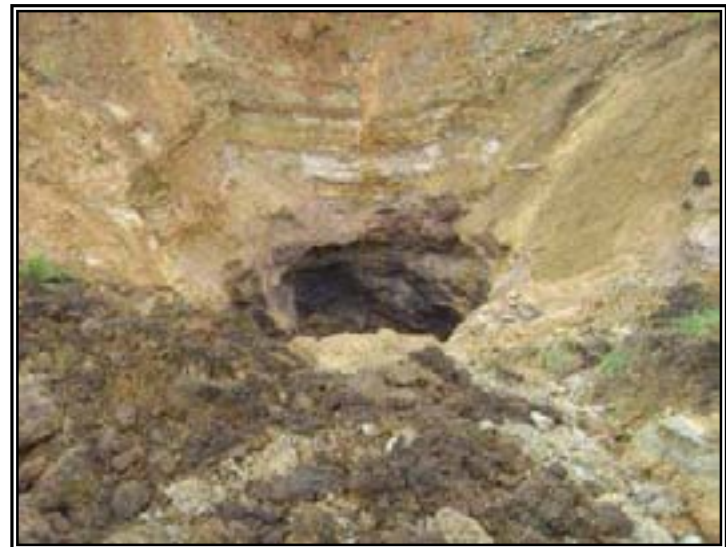
The extent of the sinkhole at Bapsfontein
