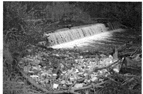
Figure 30: Vegetation and urban litter debris
